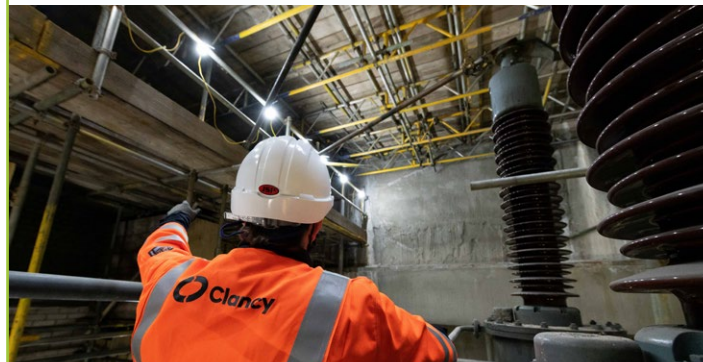
We are renewing critical substation infrastructure for UK Power Networks. A major feat of civil engineering, the project will power up the West End
